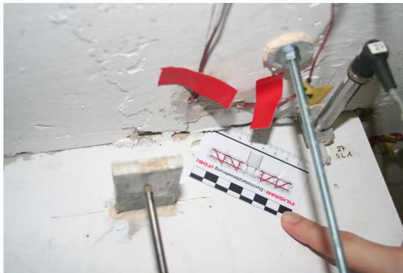
Figure 9: Test specimen FDB-E from below with a gap between column and precast slab
